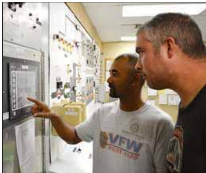
Vash Eagelson (left) shows Eric Bertrand how to operate the PLC, aka SCADA system, to include clearing alarms and viewing incoming data.
